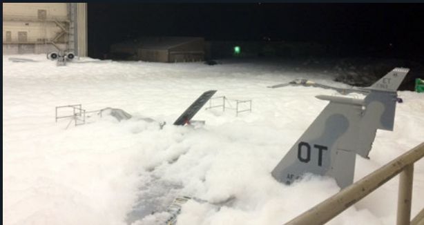
Accidental Foam Discharge at Military Hangar
